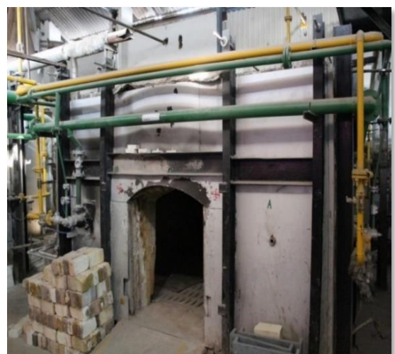
Kiln –A (4ton) – natural gas fired downdraft kiln for firing the material
